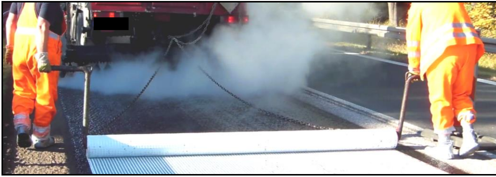
Figure 5: Installation with traverse and adjust bars directly after spraying the bond coat
